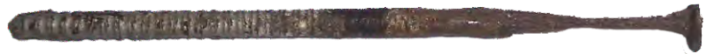
Example of a severely corroded electrogalvanized fastener. Ensure the correct fasteners are used. Corroded fasteners lead to serious sidewall system failures as well as unsightly staining.
